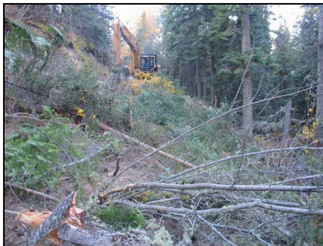
Figure 24. Recontoured site of road failure in Skidoo Creek, 2005.
