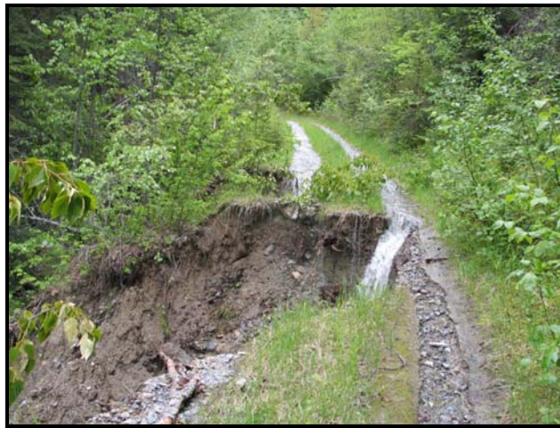
Figure 23. Road failure in Skidoo Creek, 2005
