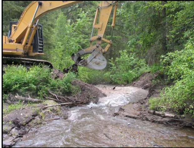
Figure 22. Site of removal of perched culvert barrier on tributary of North Fork Jocko River, 2005
