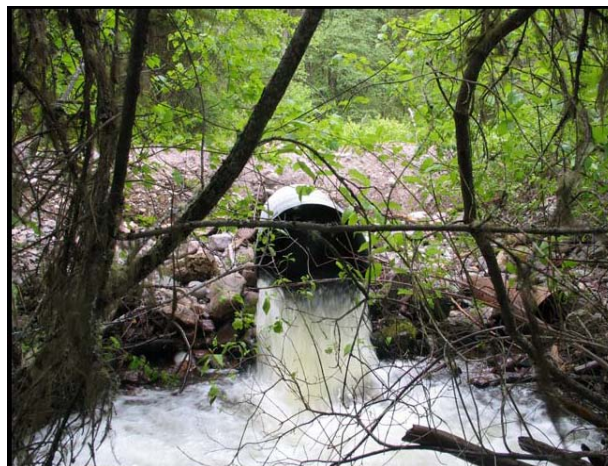
Figure 21. Perched culvert barrier on tributary of North Fork Jocko River, 2005
