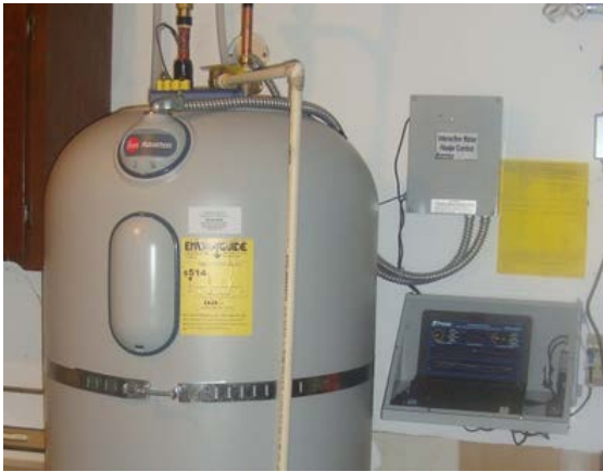
Figure: Installed 105 gallon water heater with Steffes™ mixing valve and interactive controls
