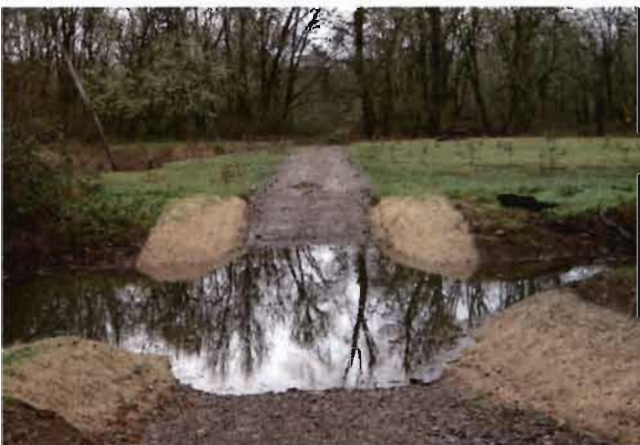
In Phase II (2006), we removed road fill in the side channel that blocked fish passage and flows like a dam. We lowered the road to the channel bed, facilitating fish passage during high flows and access for recreation and maintenance.
