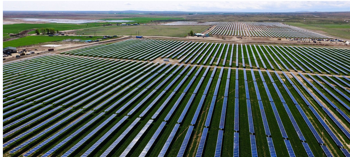
Boise City Solar, ID (40 MW) Source: Origis Energy
