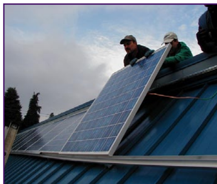
With help from Energy Trust of Oregon, this co-op grocery store installed photovoltaic solar panels and can now harness energy from the sun. (photo courtesy of Energy Trust of Oregon)
